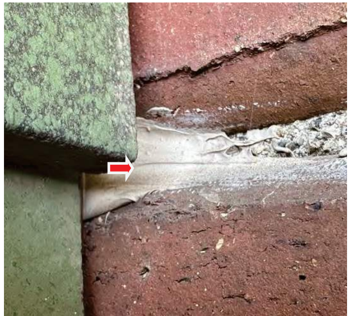
Photo 8: View of ACM exterior caulk - grey/beige, residual on Brick at NE window area. (27ABC).
