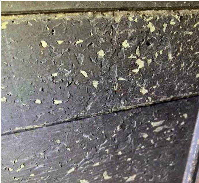
Photo 34: View of black paint on wooden loose doors stored in kitchen.
