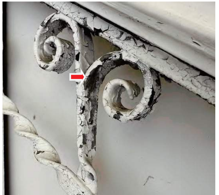
Photo 27: View of white paint on metal-central stair components.
