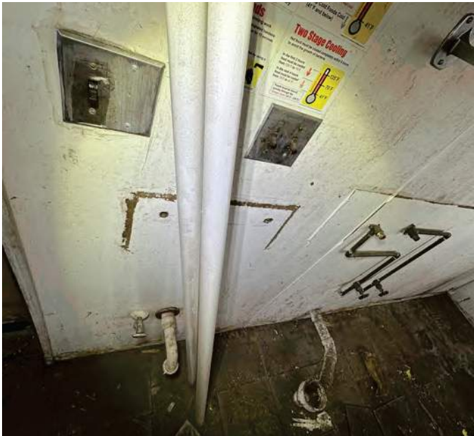
Photo 30: View of white paint on wallboard—lower level vestibules.
