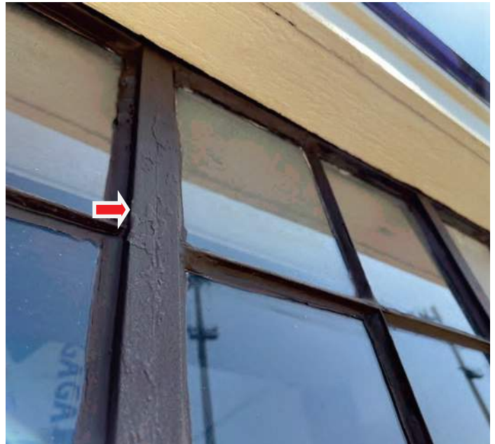
Photo 12: View of brown paint on metal - window lintel/l-beam.
