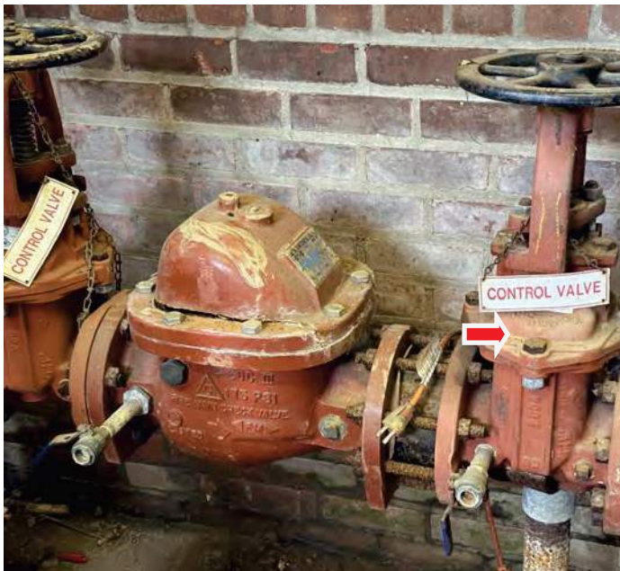
Photo 3: View of assumed ACM pipe flange gaskets.
