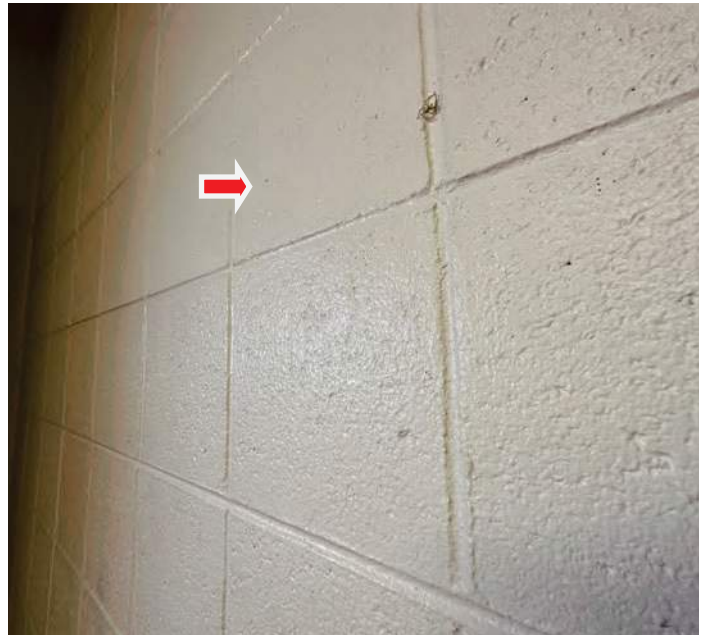
Photo 19: View of white paint on concrete.
