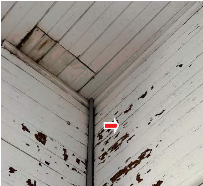
Photo 18: View of white paint on wood - upper leveling ceiling and wood walls.
