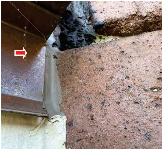
Photo 15: View of brown paint on metal - lower level window framing.
